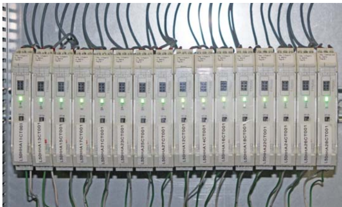
TTR200 rail mounted temperature transmitters installed in cabinet rack
