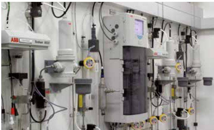
Integrated water monitoring system with the Aztec analyzer
