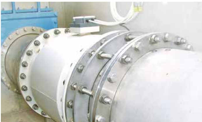
Electromagnetic flowmeter Parti-MAG on wastewater discharge pipe
