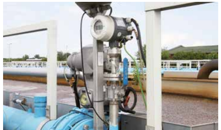
Sensyflow FMT500-IG measuring activation air in a wastewater plant
