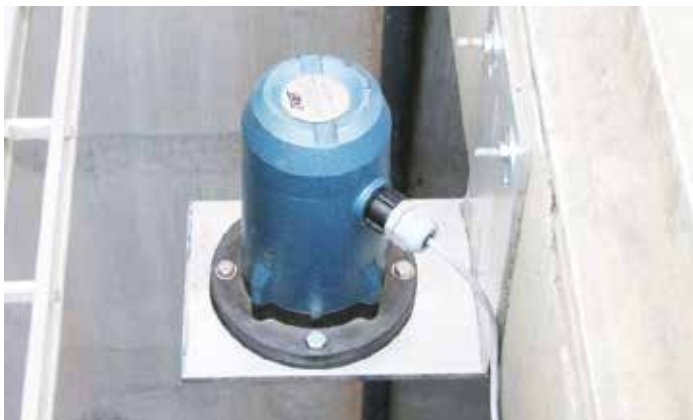
LM80 Laser transmitter in wet-well
