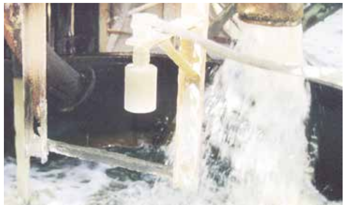
K10 ultrasonic transducer installed in sump service
