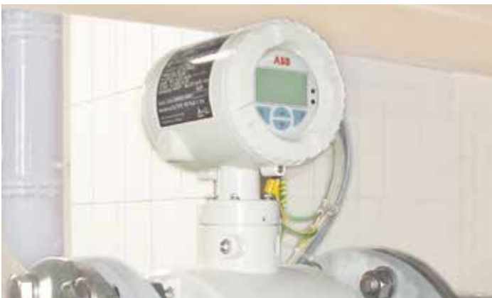
ProcessMaster installed at a filter drain pipe in a water treatment plant
